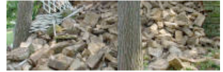
Fallen wall near the cemetery
